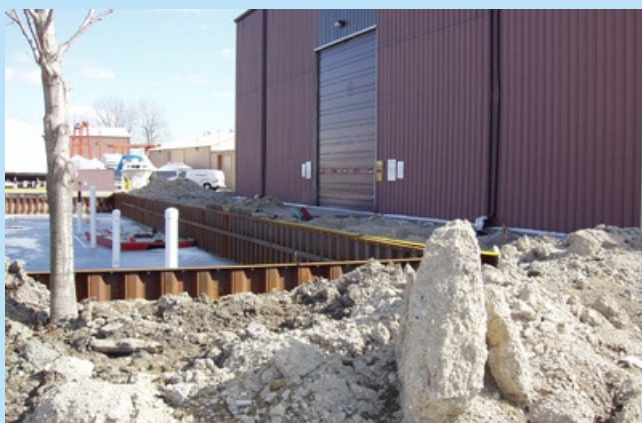
Newly replaced 150 foot section of sea wall at the rack building launch area.
