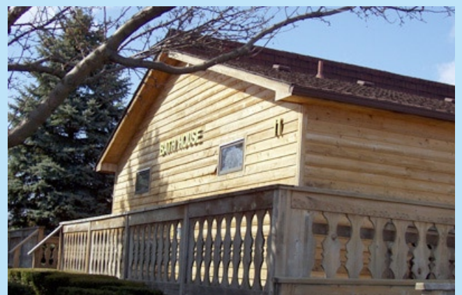
The pool bath house has been power washed and is now awaiting a new coat of solid stain
